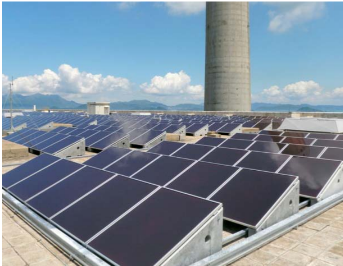
Fig. 12 – Completed PV System
