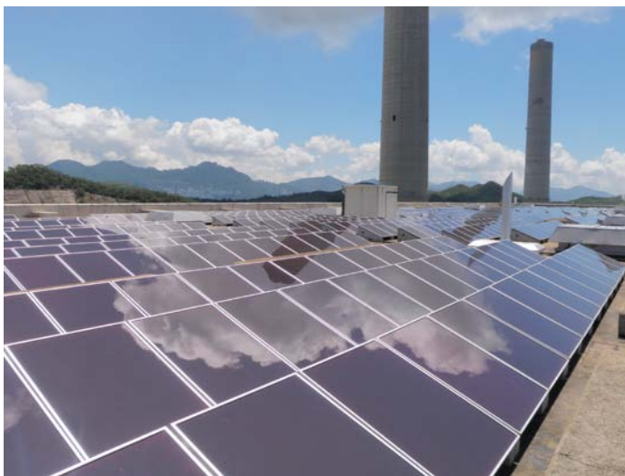
Fig. 9 - PV System at roof of Units 1-3 Boiler House
