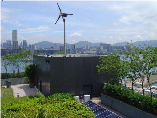
Fig. 2 – Small Scale PV System and wind turbine installed at rooftop of Marsh Road Substation
